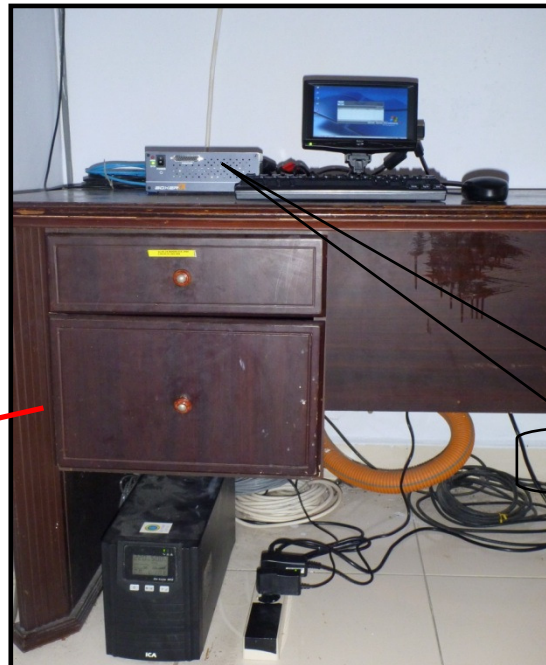
New data transfer system
