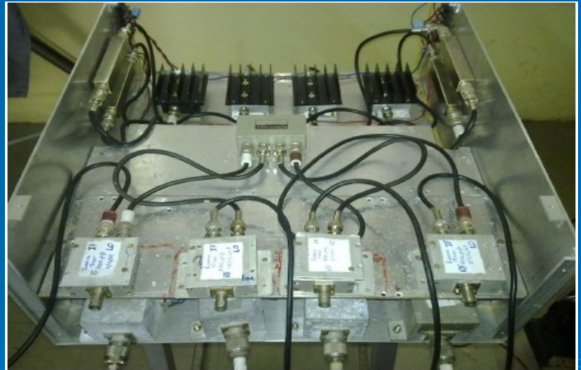
Figure 6.5: New back-end receiver system
