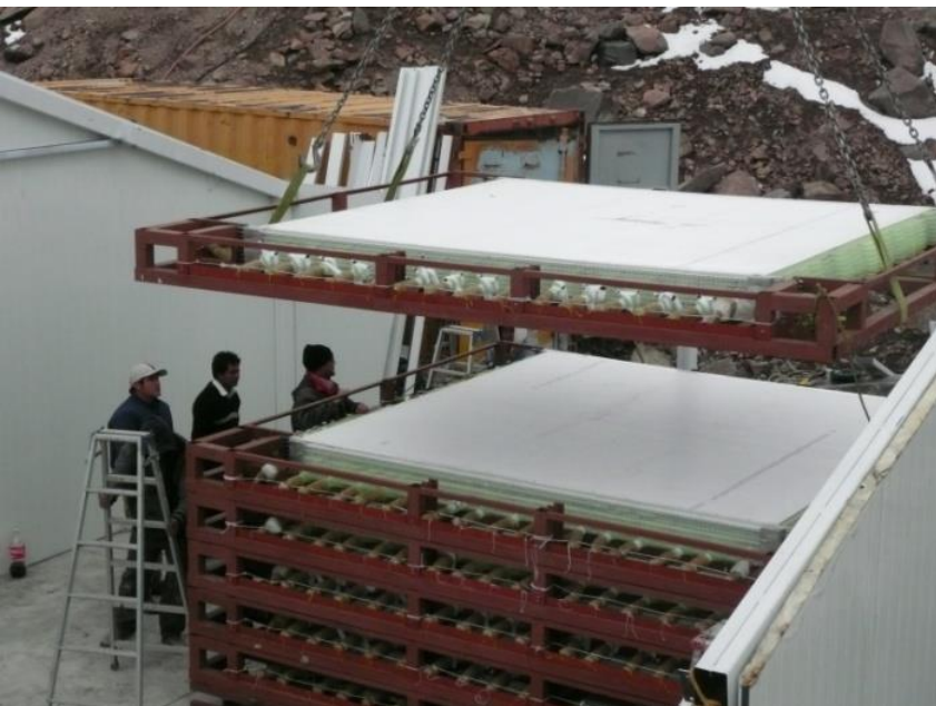
Installed in April, 2013
