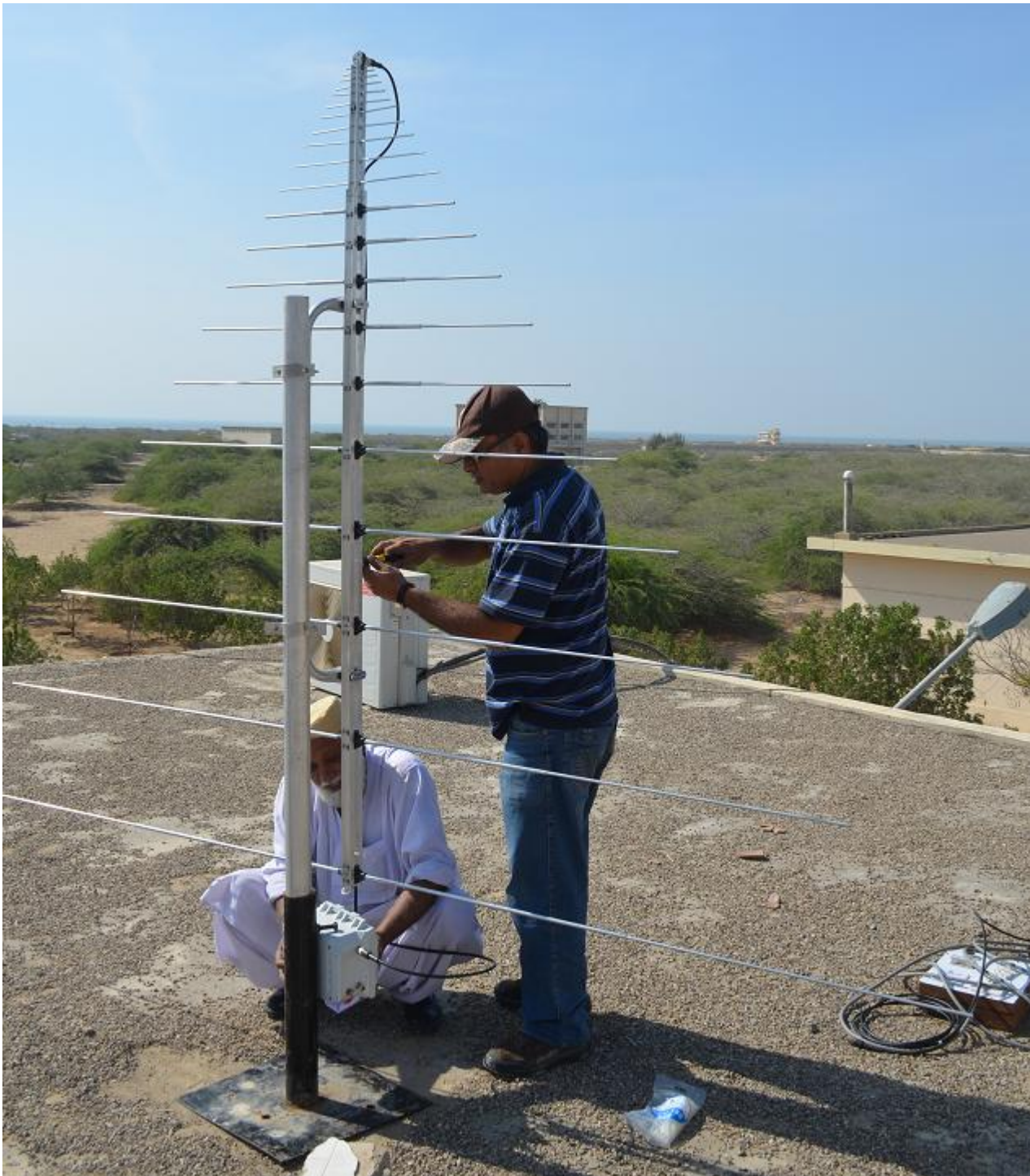
Fig 4: Installation of the LPDA on the roof of the observatory. The focal plane unit containing low noise amplifier was produced by W. Reeve in Anchorage, Alaska/USA.
