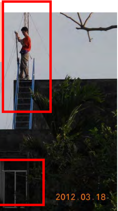
Mr Imajo installs our GPS antenna at the highest point of the observatory.
