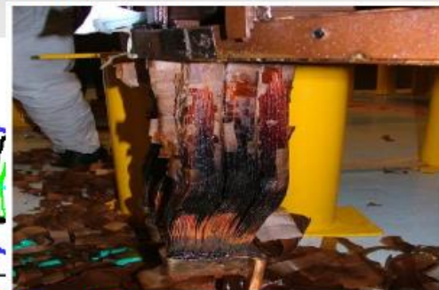
Station 3 Transformer 6 LV exit lead overheating
