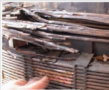
Station 4 Transformer 6 HV winding failure
