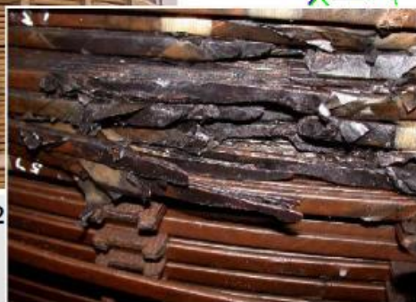
Station 3 Gen Transformer 4 damage
