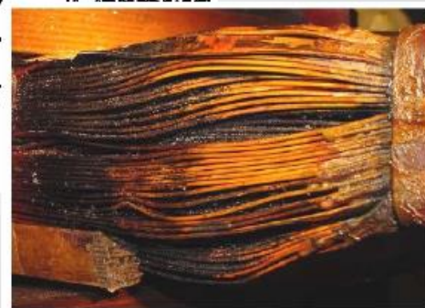
Station 3 Gen. Transformer 5 overheating
